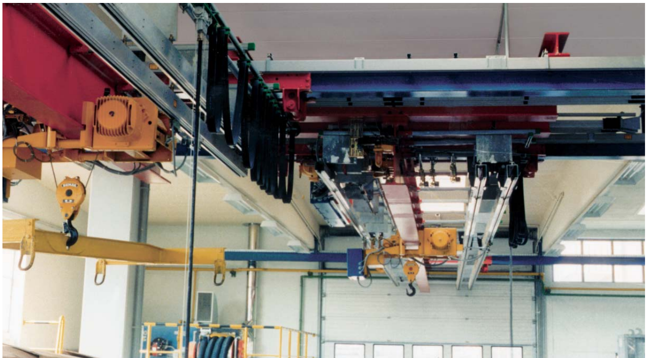
Aluminium enclosed conductor system on crane bridge.
